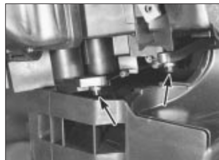
8.6c Control cable connections to flap valves at heater distribution box unit (arrowed)
